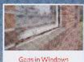
Gaps in Windows or Door Frames
