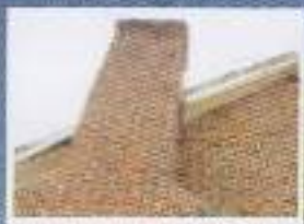
Leaning or Tilting Chimney
