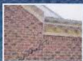
Exterior Wall Cracks
