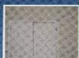
Interior Wall Cracks
